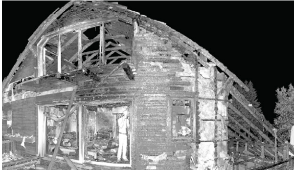
3D point cloud of a burnt restaurant
